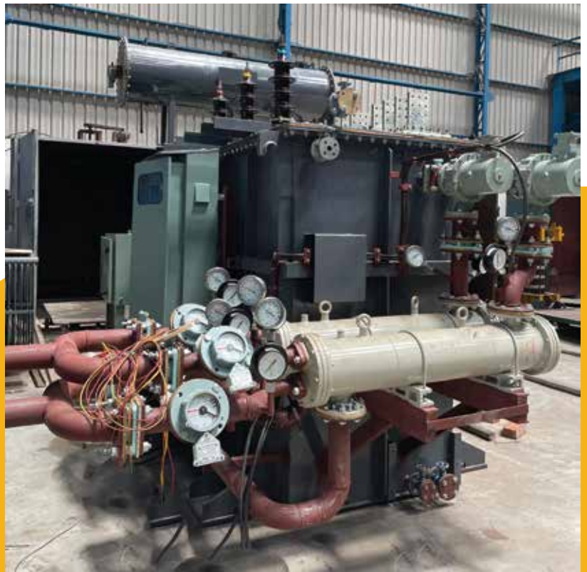
4MVA 33KV LRF TRANSFORMER OF DTPL, GUJARAT
