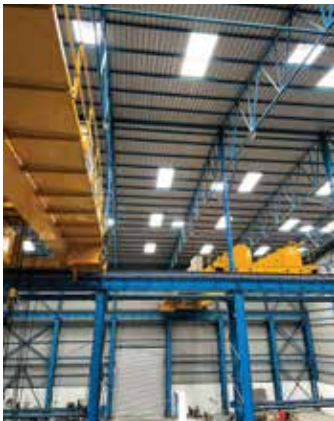
60MT (30MTX2) EOT CRANE BAY'S
