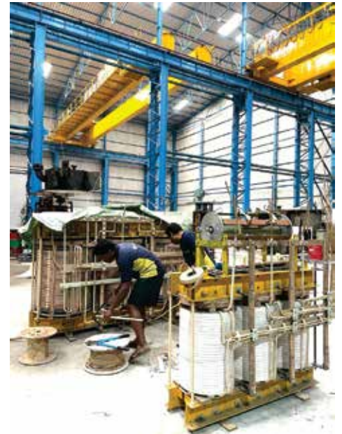
ACTIVE PART OF TRANSFORMER AND REACTOR
