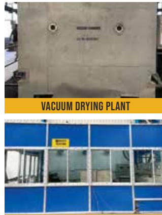
COMPLETE TRANSFORMER TESTING FACILITY
